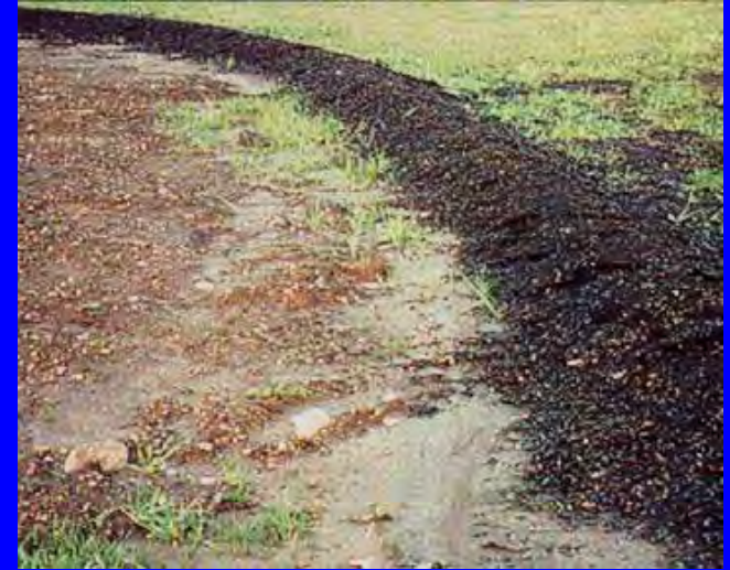
Berms instead of silt fence
